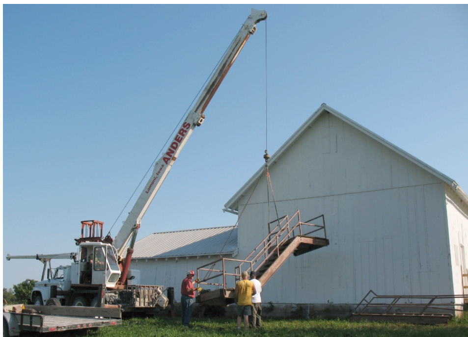
Installing a historic fire escape was a crowning touch for the barn.
