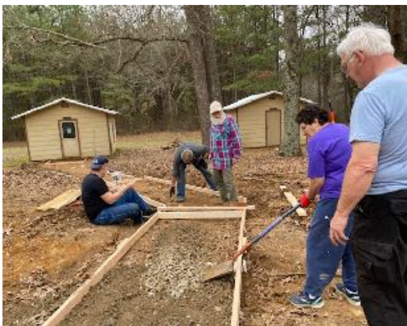
RVA workers helped replace a walkway between Liberty Hall and Spurrier School.
